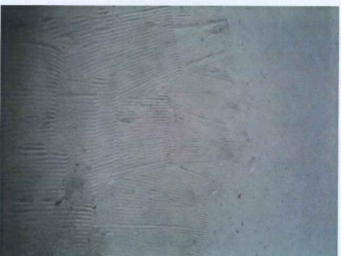
Image 6: Unacceptable rake job.
